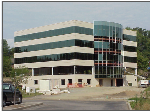
Franklin Park Corporate Office Building during the precast erection phase of construction.
